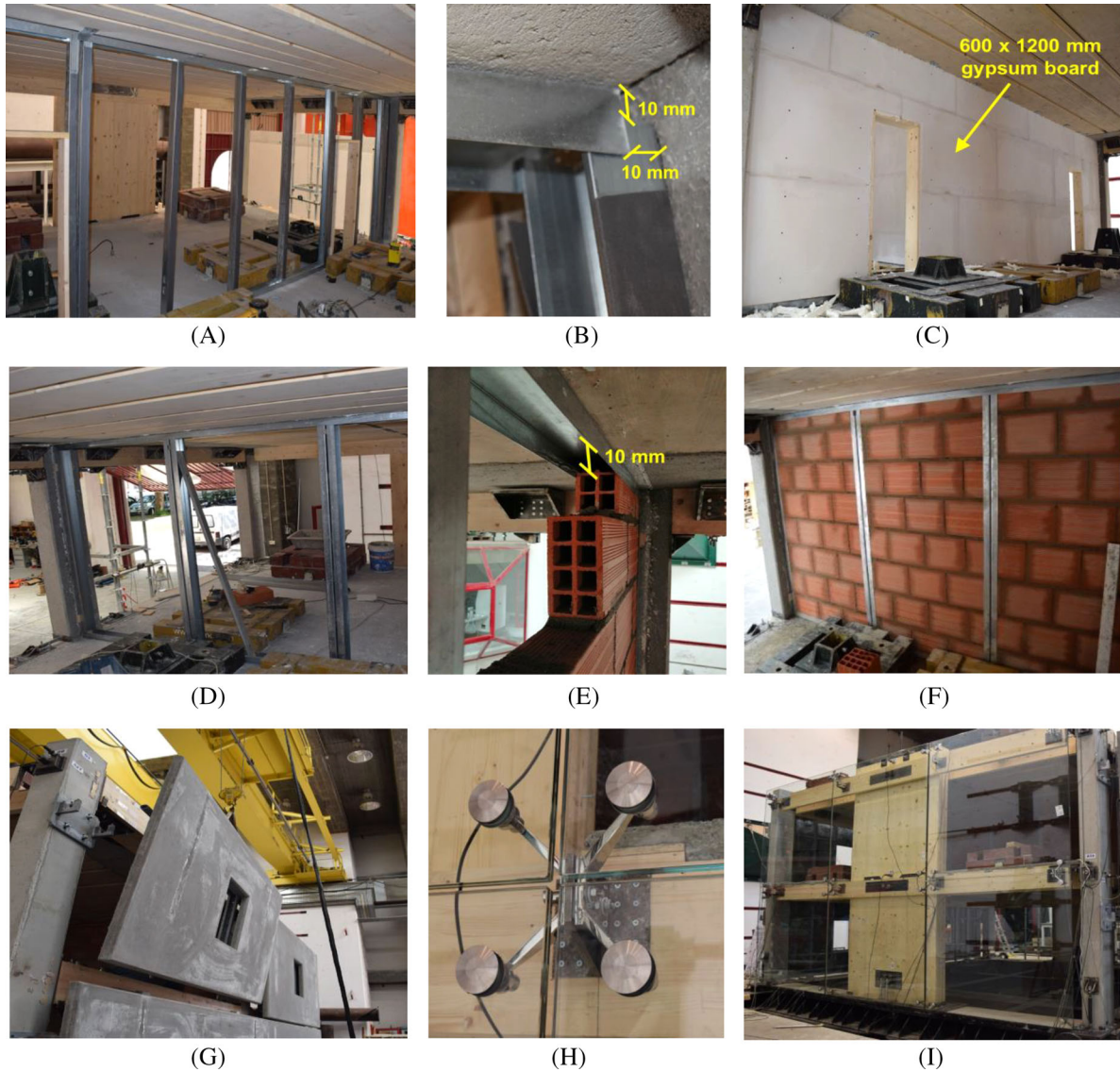
FIGURE 9 Construction/assembly of: (A–C) the fiber-reinforced ceramic gypsum partition; (D–F) the low damage masonry infill wall; (G) the GFRC facades; (H, I) the spider glazing facades.
