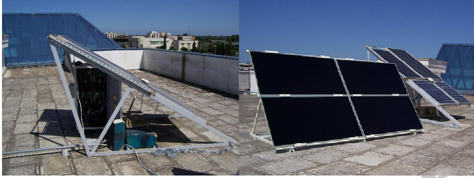
Figure 3. View of thin-film CdTe PV modules located on the Dept lab roof
